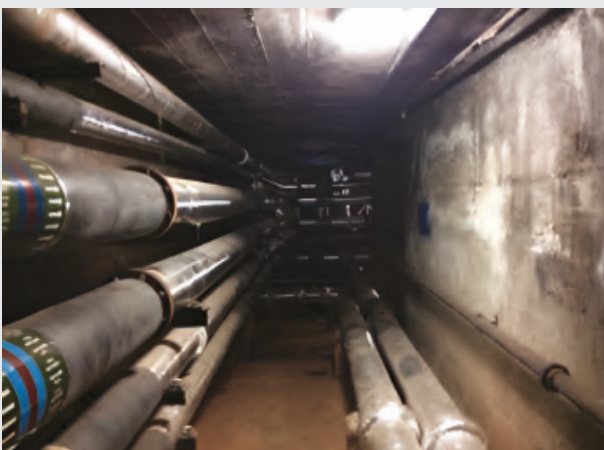
Fig 5. LTHW pipework is routed via services tunnels to each individual building.
