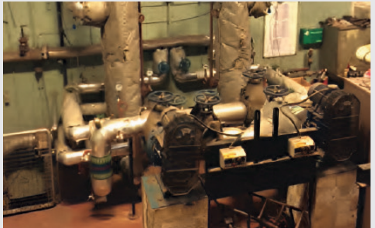
Fig 4. Two Pullen belt driven circulating pumps with two Steam fed vertical heat exchangers.
