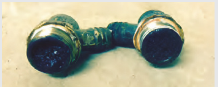
Fig 6. Two 1/2" Brass DOCs. These were removed from a fouled pipe during a clean-up operation and show the effects of corrosion debris. Ultra fine particles that are capable of passing through system strainers will still settle out in low flow parts of a system.
