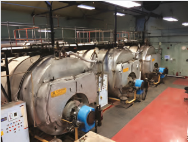
Fig 3. No Riley steam boilers installed in 1960s.
